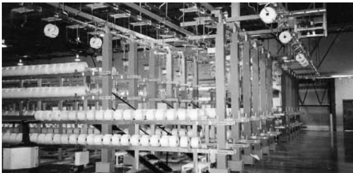
Fig. 66 Package pre-storing conveyors
